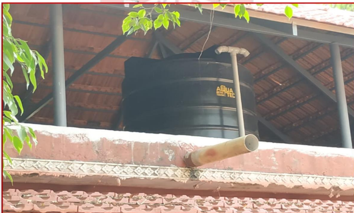
Water Tank Protected from Direct Sunlight
